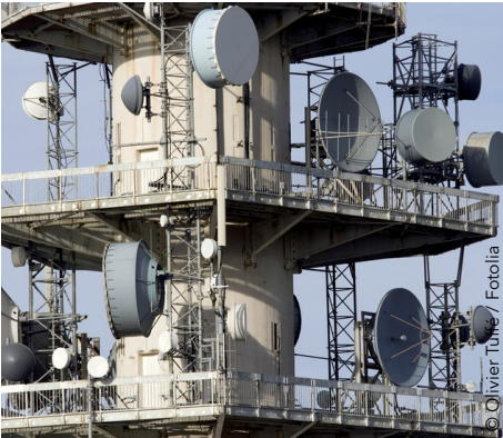
Telecom - Data infrastructure
