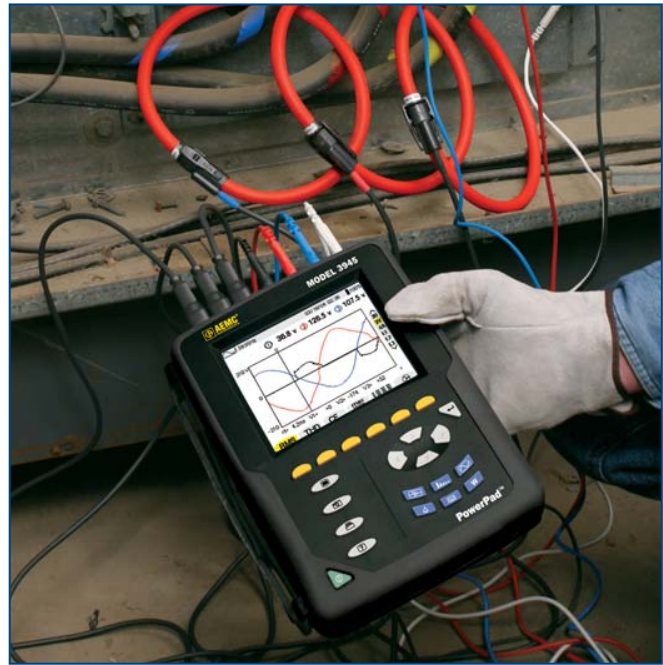
Power quality analysis on a three-phase panel using the AmpFlex™ flexible current probes.
