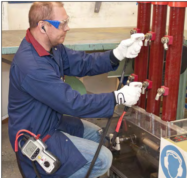
Hold probes / attach Kelvin clamps to CB and press trig / TEST button. A signal indicates whether test was pass or fail and result is logged in unit for later dump to PC.
