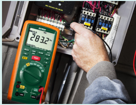
Voltage check on motor starter
