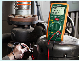
Insulation test on pump motor
