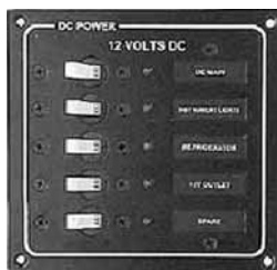
DC Distribution Panel
