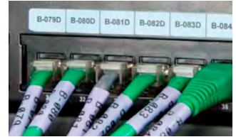
Patch Panel Labels
