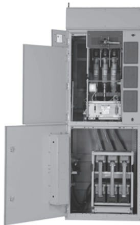
AMPGARD IT. Soft Start (Doors Open)
