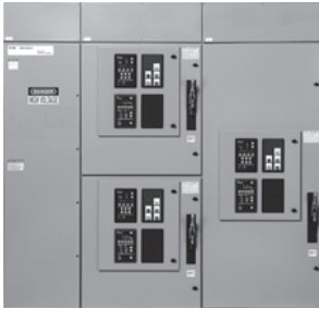
Next Generation AMPGARD Lineup— Front View
