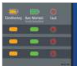
Battery fault detection LEDs
