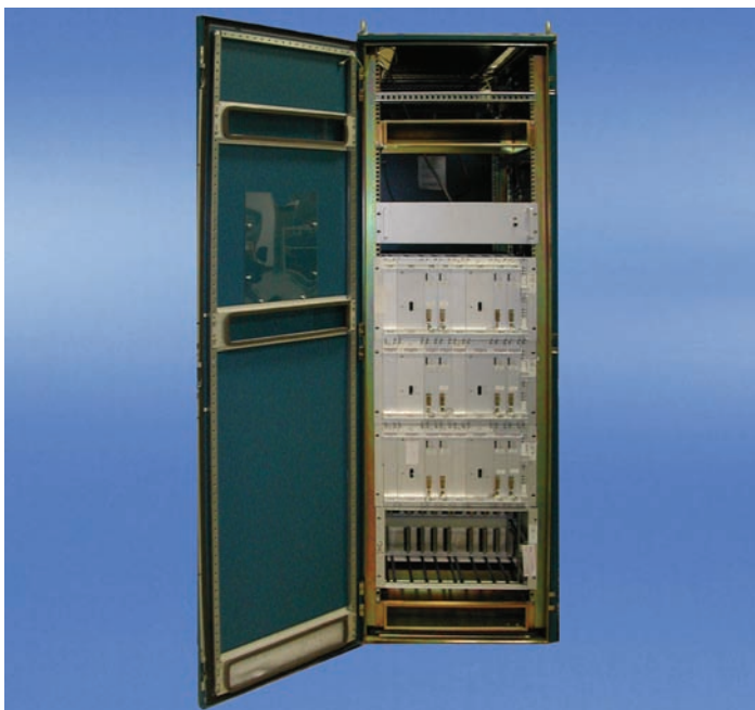
Application: Control system
